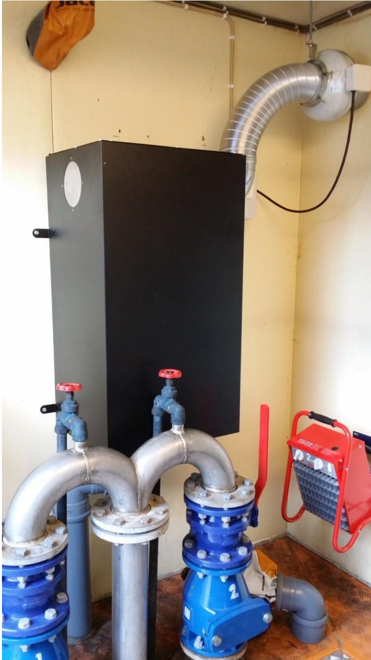
Figur 1: BlackBox smart installerad i en pumpstation.
